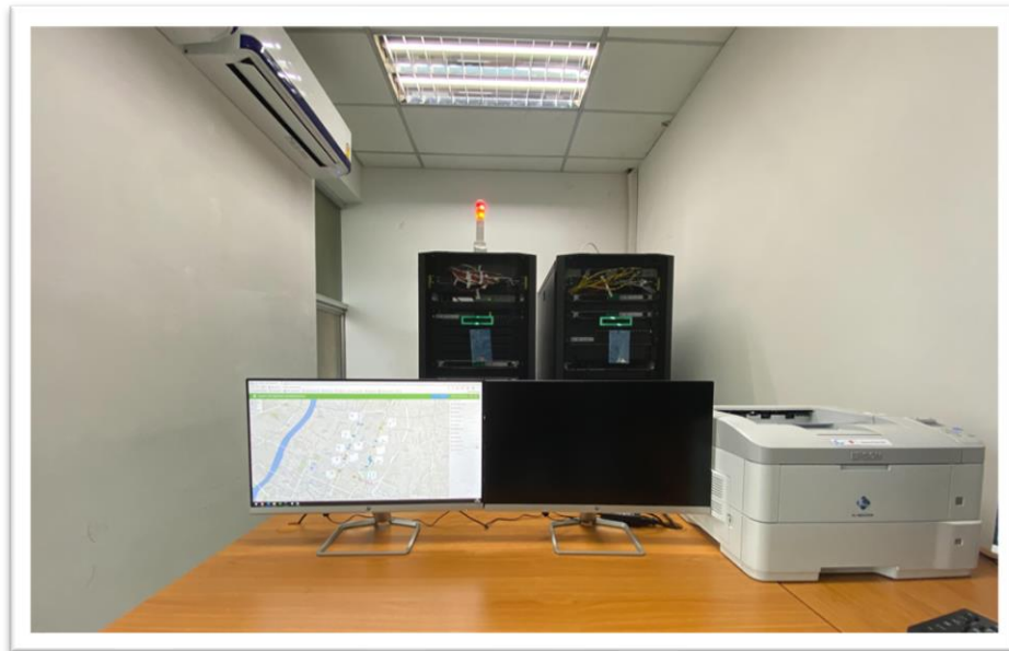
Control Center at TTD
