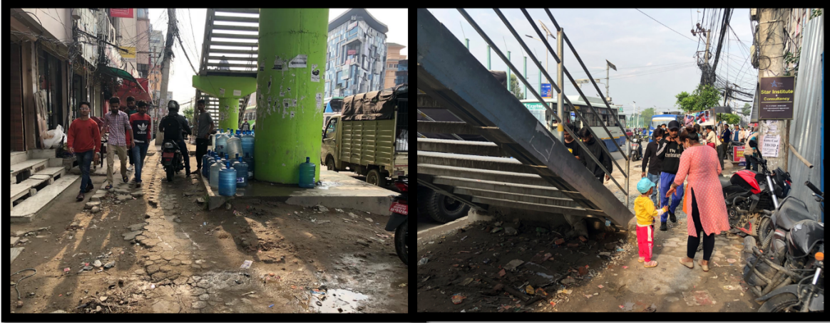
Figure: Sidewalks require reconstruction to accommodate the vulnerable users
